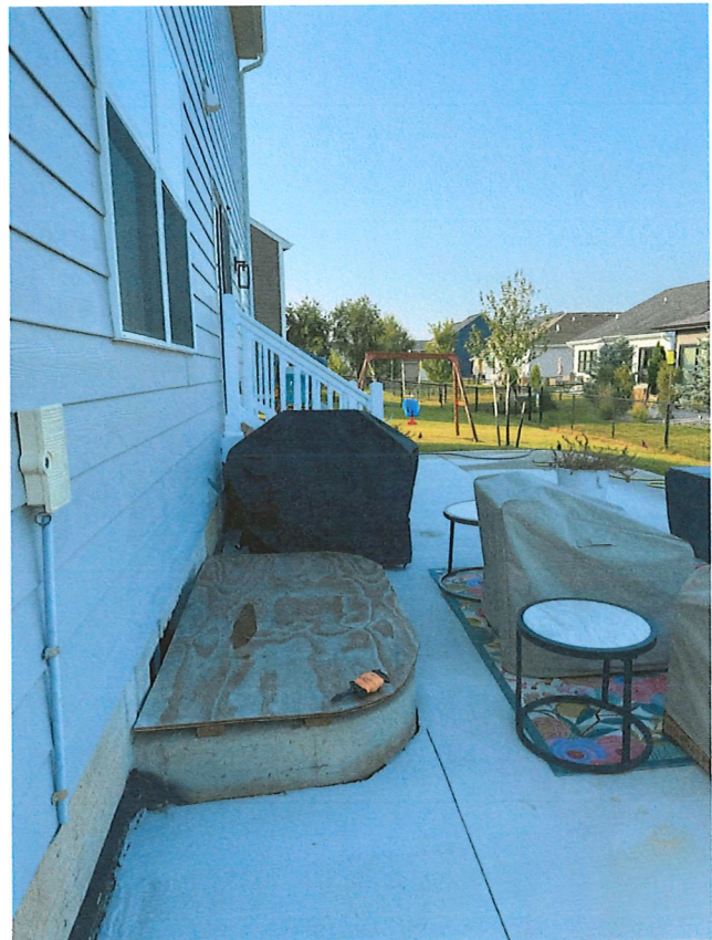
Almost 4 ft depth window wells (42-inch) reduce usable area and create a play hazard, further limiting locations for shade.
