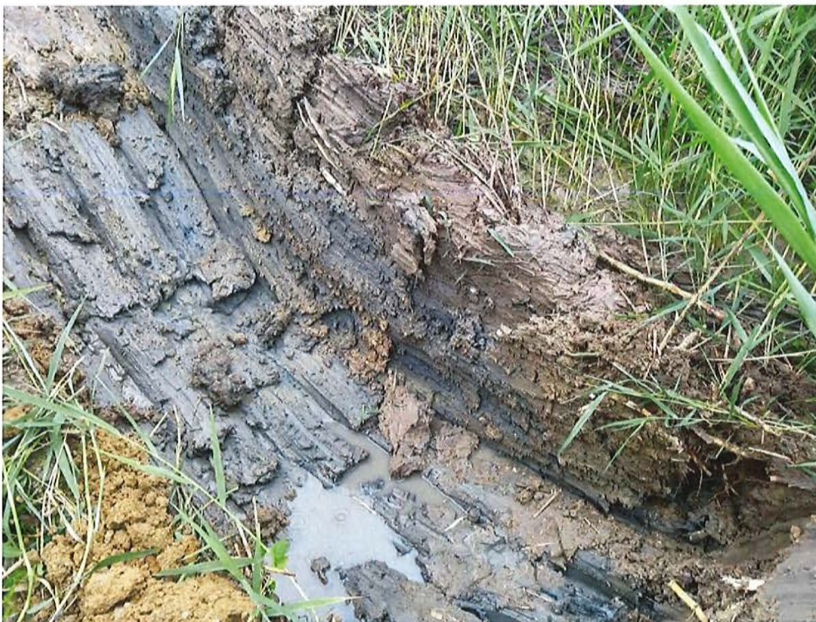
Photo No. 1 - Very Moist and Soft Unstable/Unsuitable Soils Present in Upper Portion of Swale
